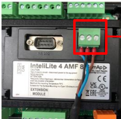
MAIN SCO 11 communication wire
