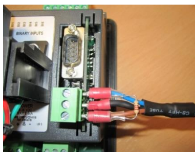
MAIN SCO 10 communication wire end
